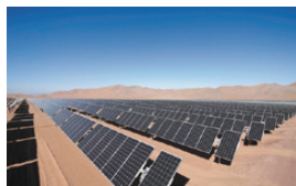
Mogalakwena solar PV plant
