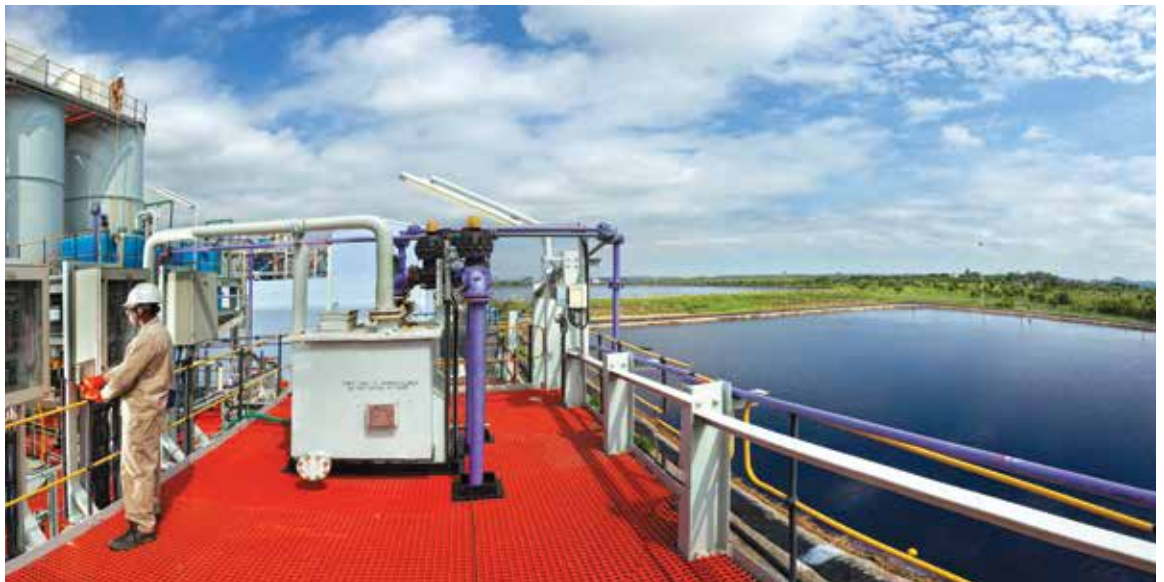
Image The evaporation plant at Precious Metals Refinery.
