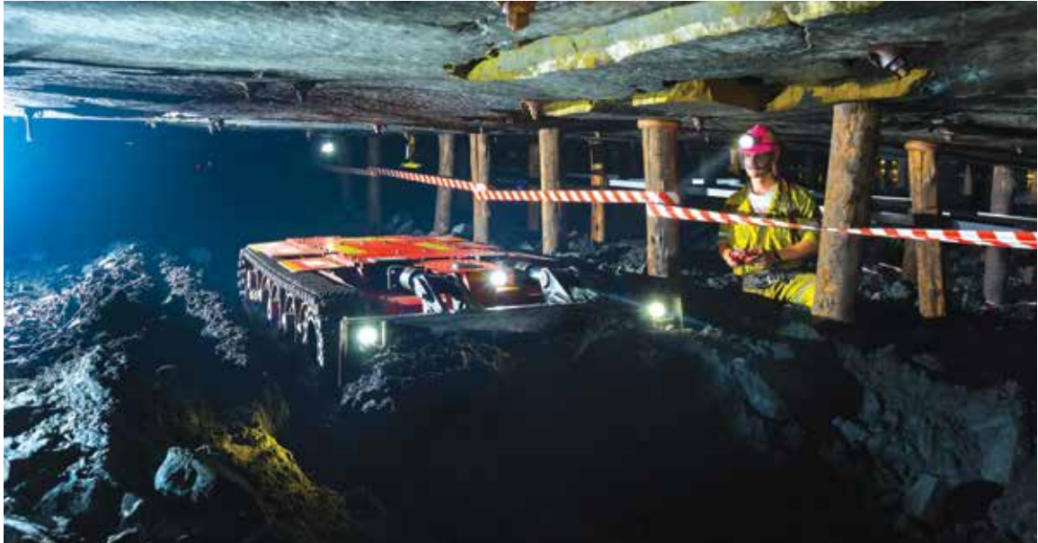
Image Conrad Van Zyl operates an ultra-low profile remote operated dozer at Bathopele Mine.
