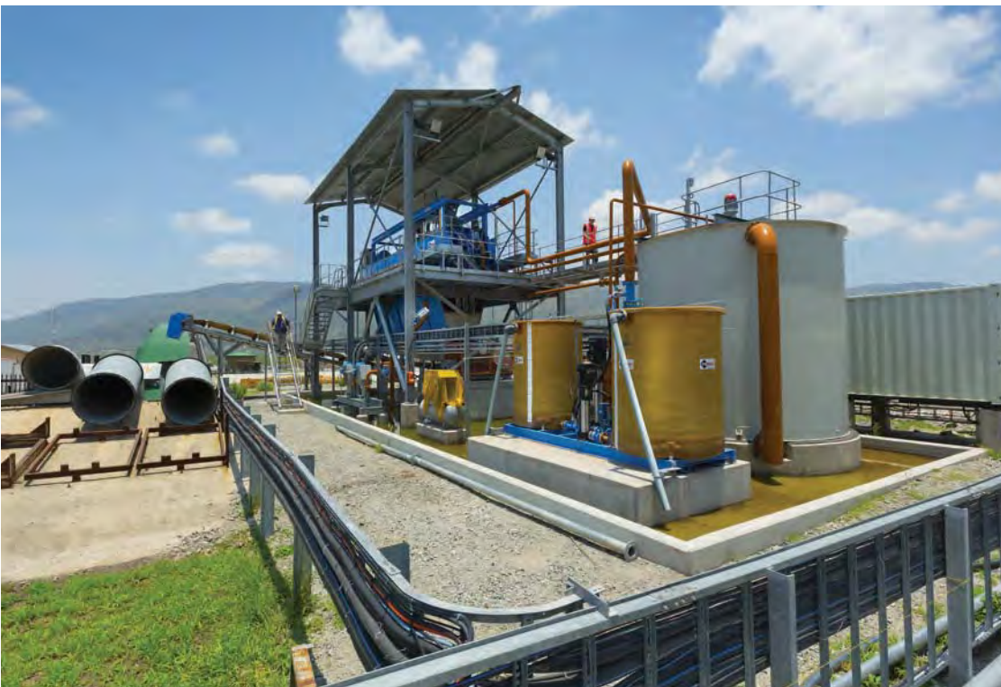
Filter press unit at Twickenham Mine used to reduce sediment in return water.
