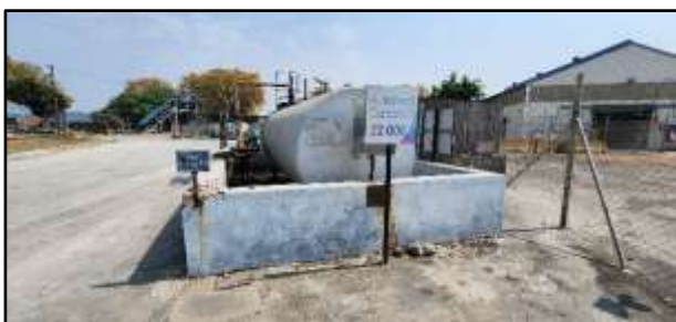
Picture 13: Diesel storage bay (1)
