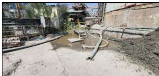
Picture 8: Leaking process water
