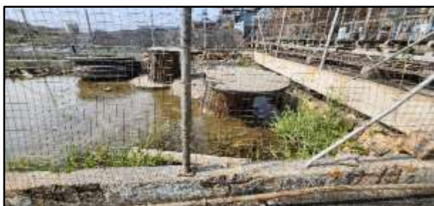
Picture 7: Pooling water
