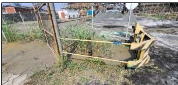
Picture 5: Silted trench
