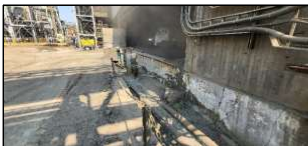
Picture 3: Damaged trench
