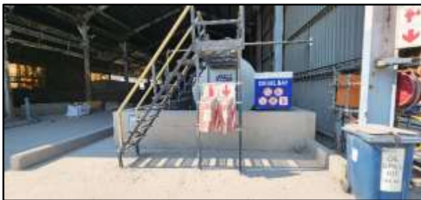
Picture 11: Bunded Diesel storage tank
