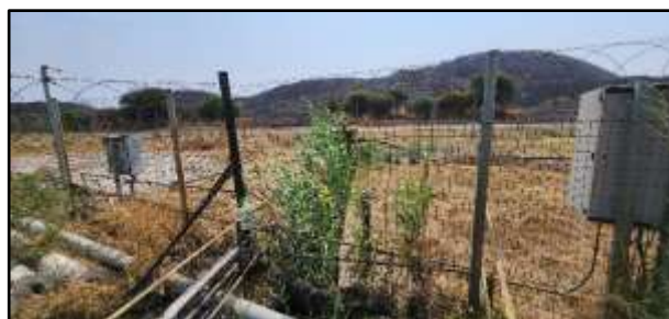
Picture 6: Silted trench with vegetation growth
