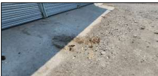
Picture 35: Oil spillage at oil store.
