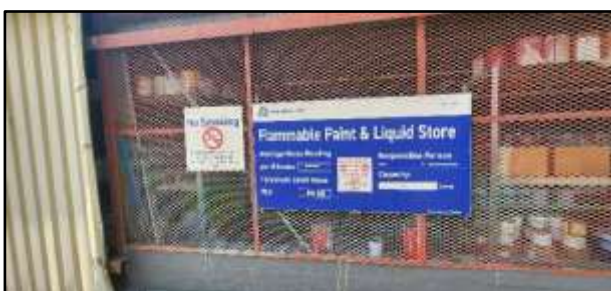
Picture 15: Bunded paint stores
