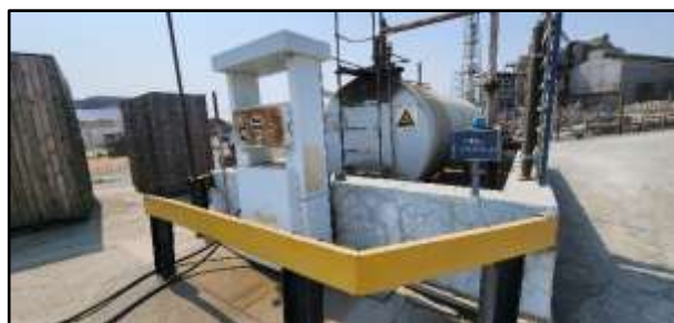
Picture 14: Diesel storage bay (2)
