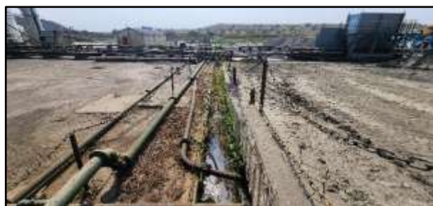
Picture 4: Silted trench with vegetation growth
