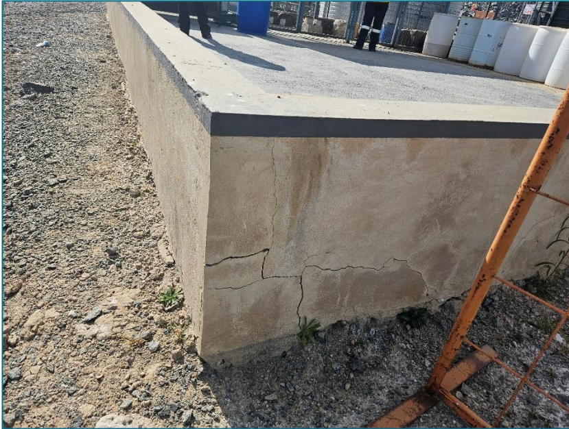
Figure 3.2-7: HCS bund wall cracks
